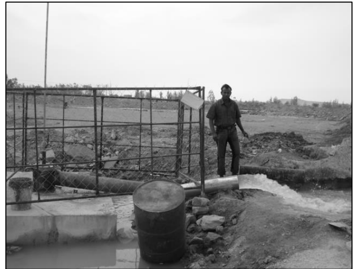
Figure 7: Controlling the discharging waters
